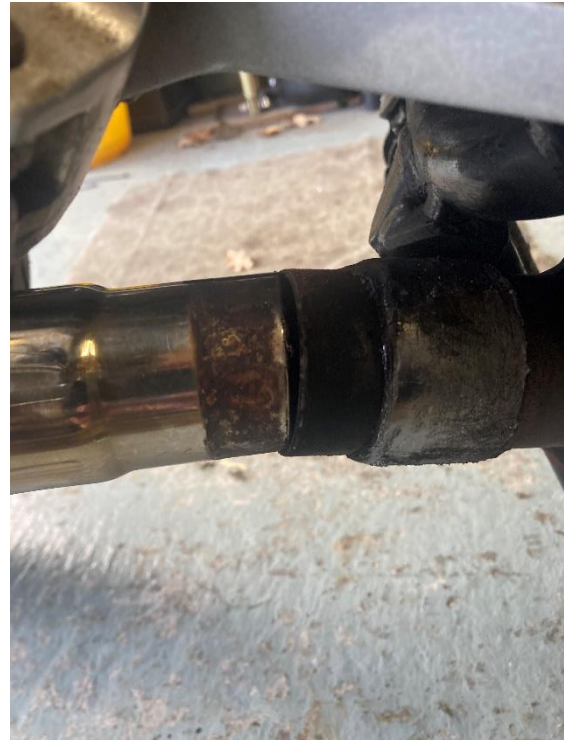
Pipes that didn't fit
